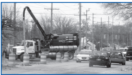
Workman continue to install new sewer lines under Kennedy Avenue near LaPorte Street.
